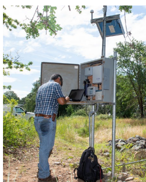
Above: A water resources technician with California Department of Water Resources, works at the station house of the newly installed North Honcut Stream Gage on Honcut Creek in Butte County, California.
