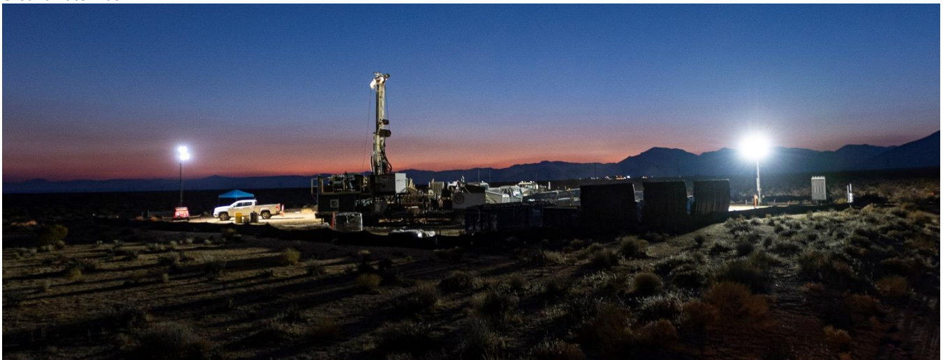
Photo 1: DWR Staff and Contractors Work to install a New Well to Monitor Groundwater Conditions in the Indian Wells Valley Groundwater Basin.
