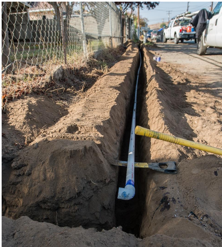
Photo 3: New Water Lines are Installed in Tulare County to Connect Impacted Domestic Well Owners to a New Municipal Water System.
