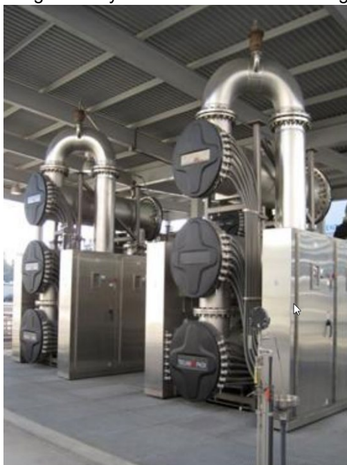
Figure MM05-1. Advanced Water Purification Facility UV/AOP System. (Orange County Water District, 2021a).
